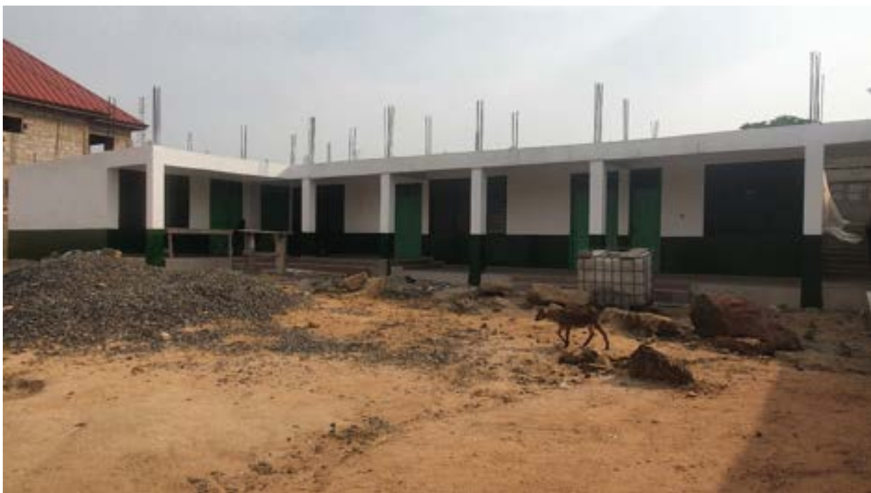
CONSTRUCTION OF 3-UNIT CLASSROOM BLOCK AT IBAADU RAHMAN ISLAMIC CENTRE LASHIBI (DACF)
