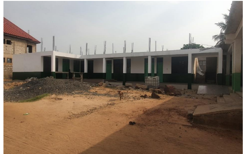
CONSTRUCTION OF 3-UNIT CLASSROOM BLOCK AT IBAADU RAHMAN ISLAMIC CENTRE LAASHIBI (DACF)
